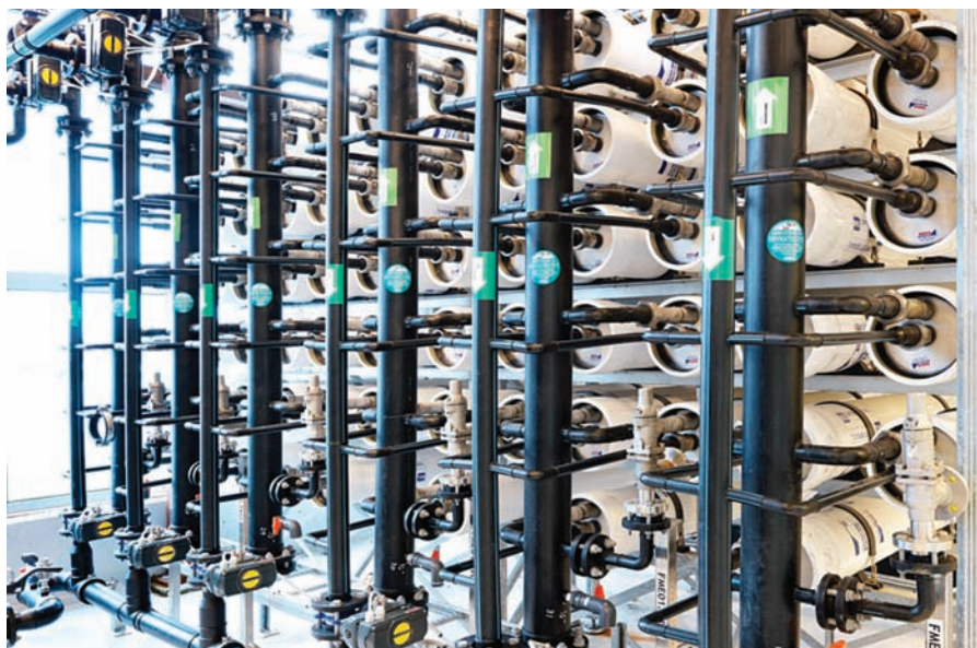
World first: membranes inside pressure vessels are key to the operation of Tofte's facility
